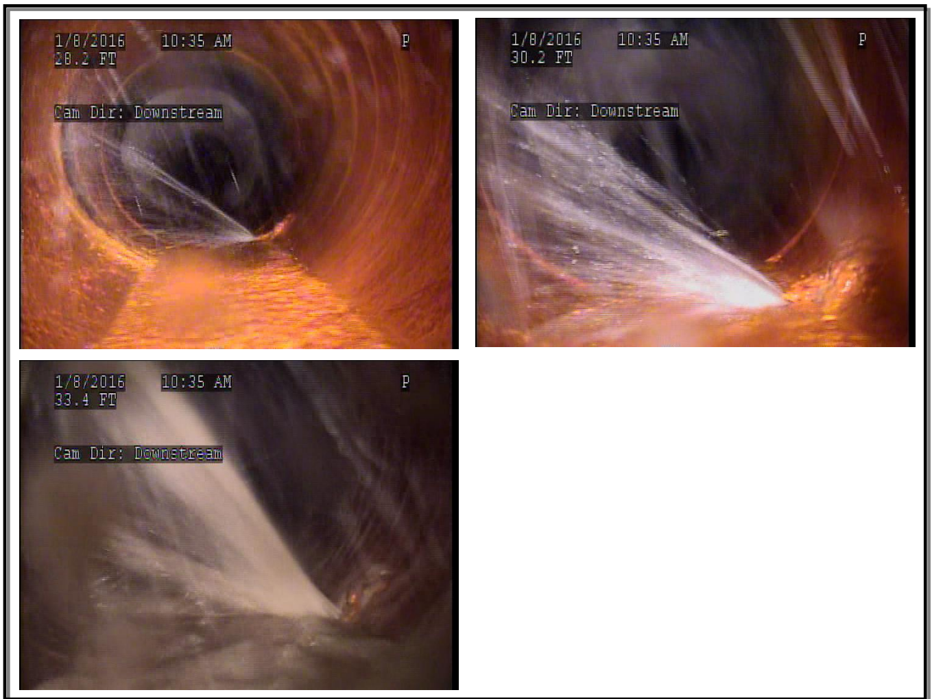
Figure 3: 2016 Gusher (MH 37 – MH 38)
