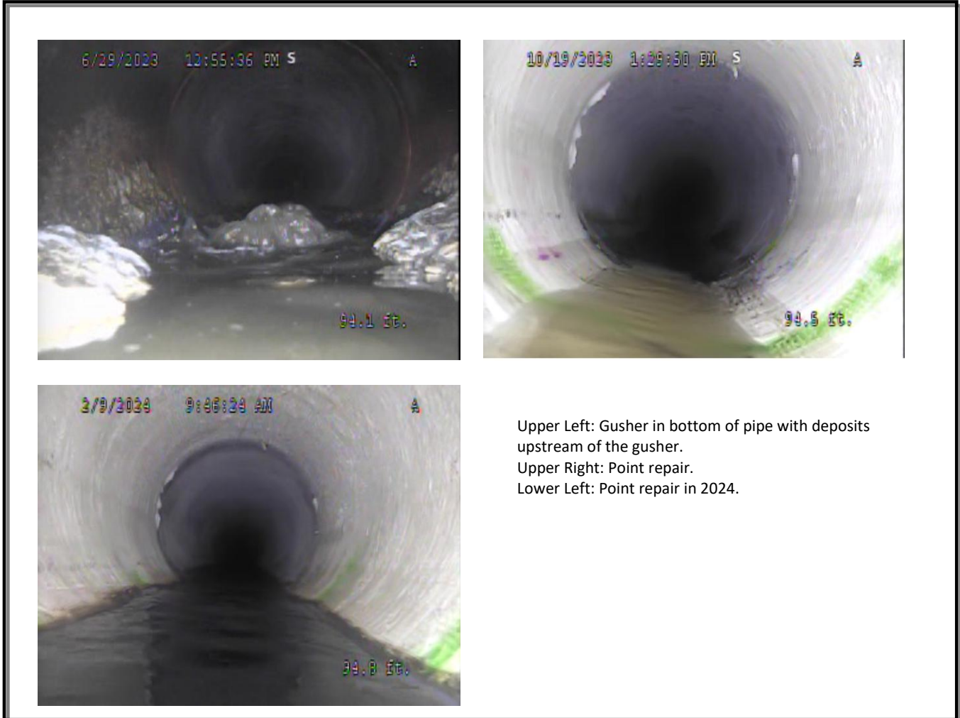
Figure 5: 2023 gusher (MH 35 - MH 36) and point repair
