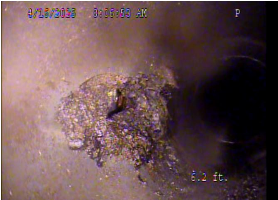
Asset ID: 09LN000979062061 (Hole void visible)
