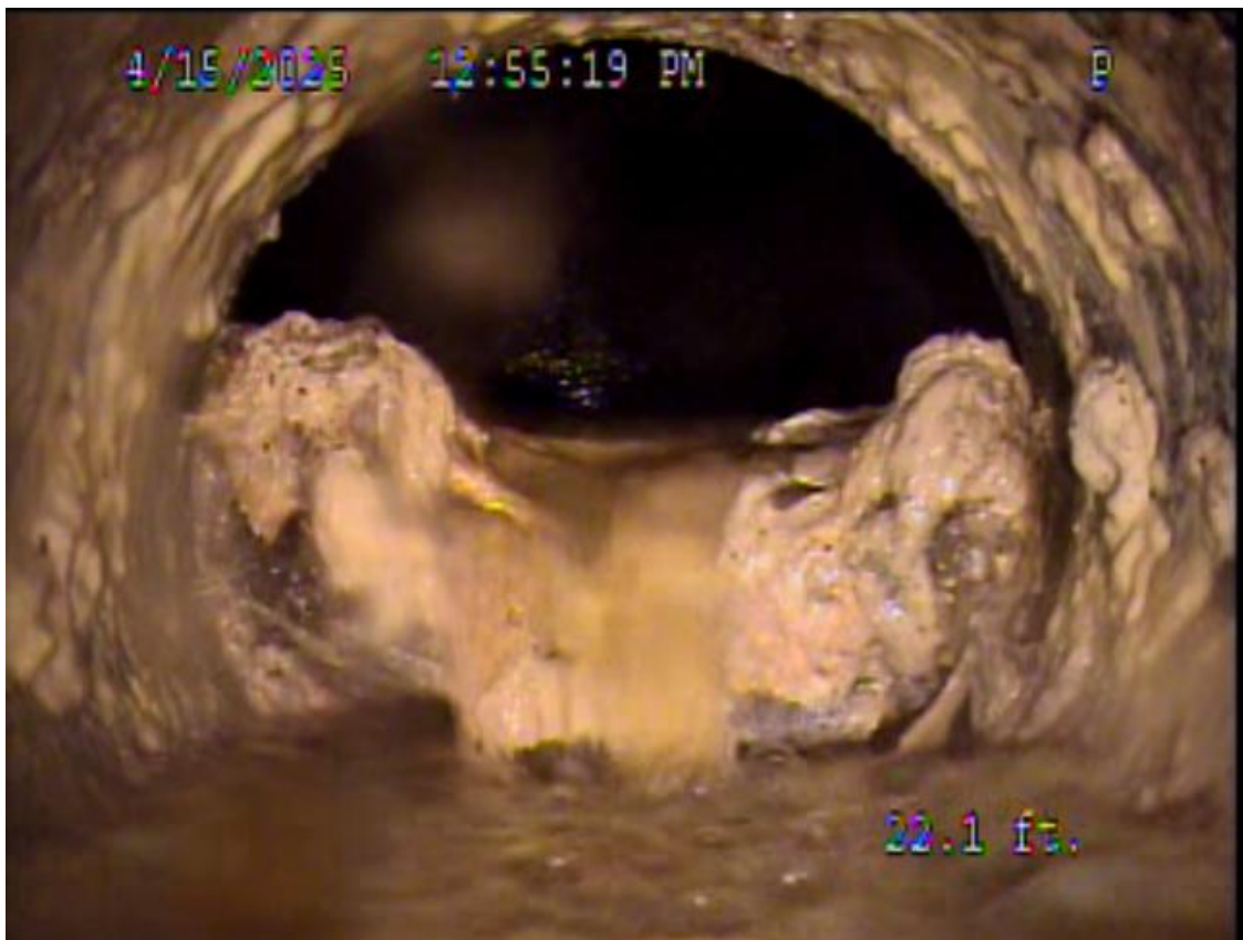
Asset ID: 09LN000978060053 (Obstruction)
