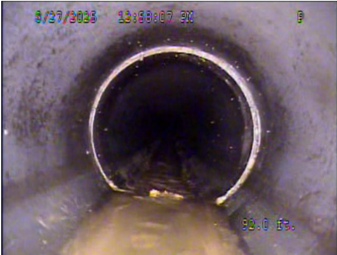
Asset ID: 09LN000979064063 (Joint separated)
