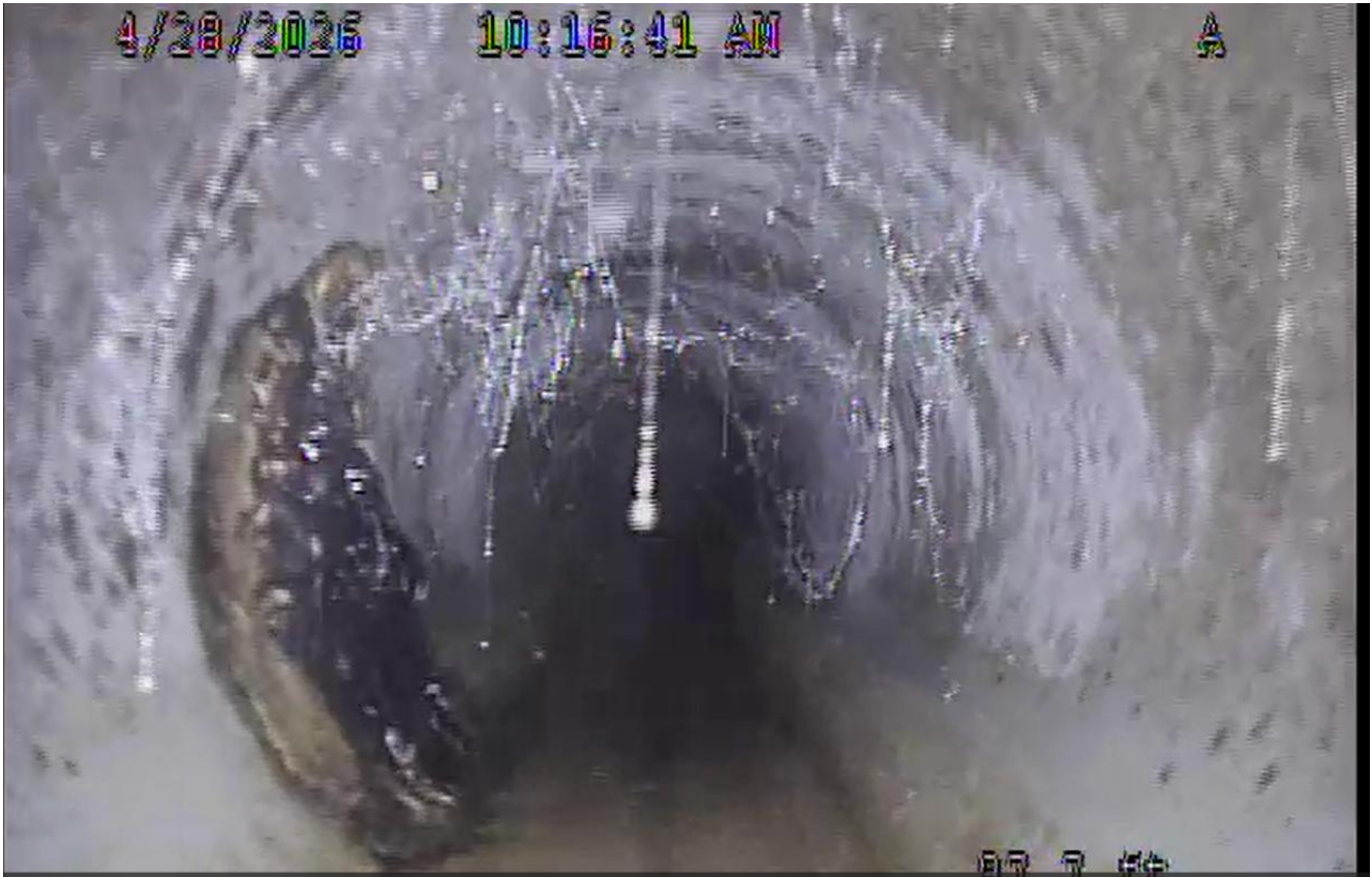
Asset ID: 09LN001411049046 (Encrustation)
