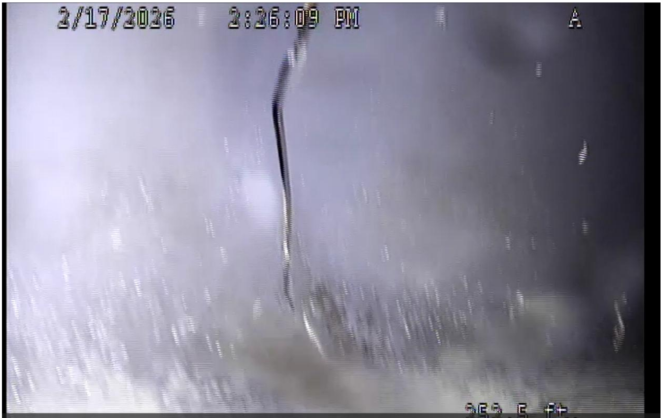
Asset ID: 09LN000977008007 (Vertical crack)
