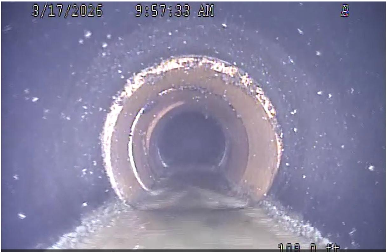
Asset ID: 09LN000978044043 (Offset joint)
