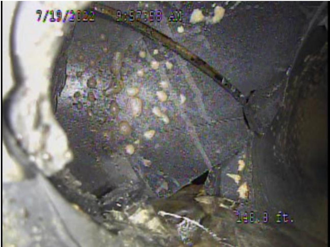
Asset ID: 09LN001147041019 (I&I – Broken pipe)
