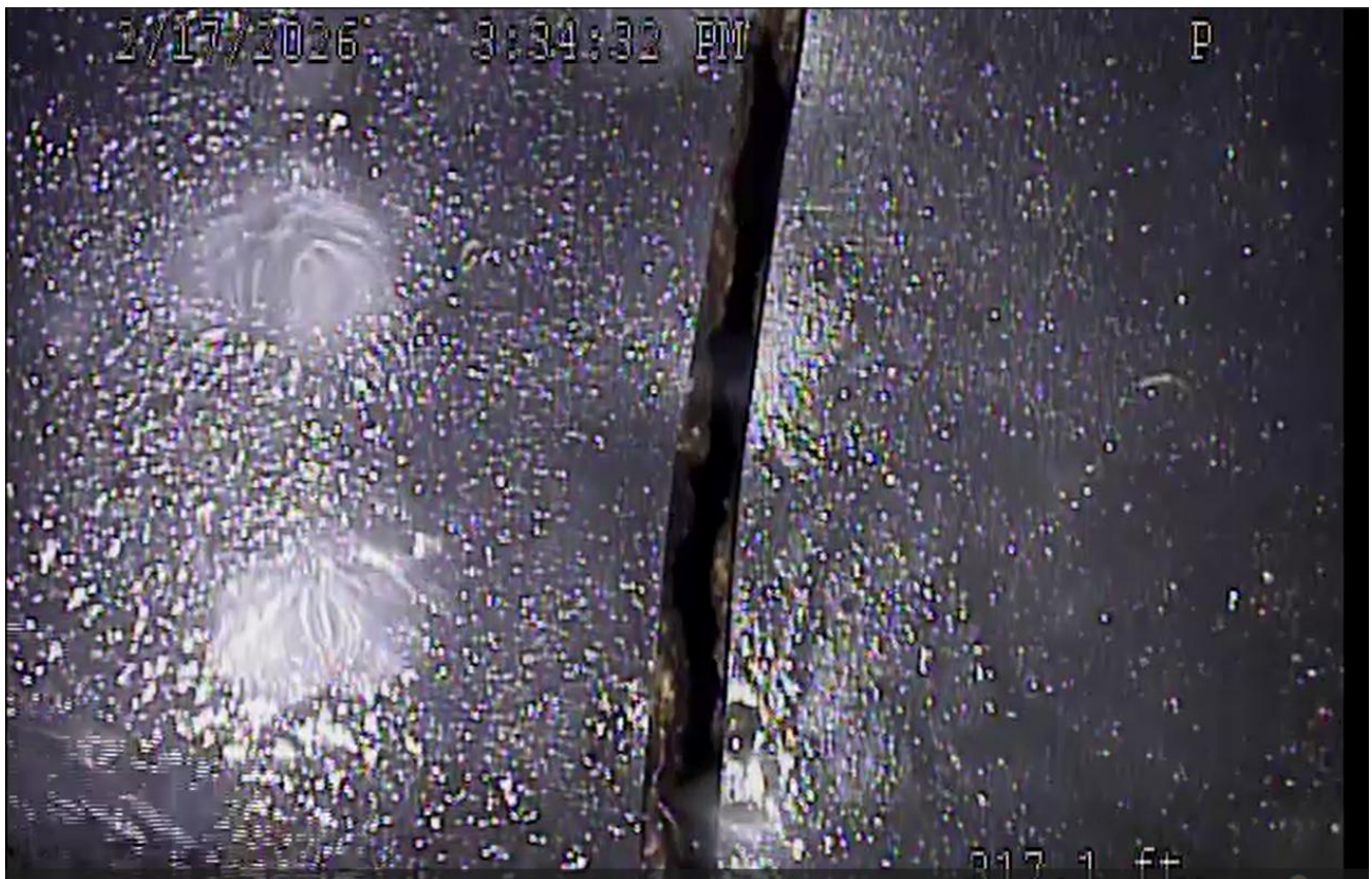
Asset ID: 09LN000977005004 (Vertical crack)
