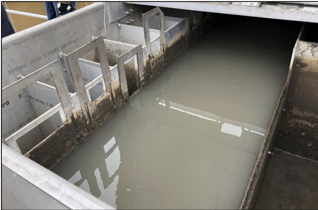
Figure 2-2: Influent Distribution Box
