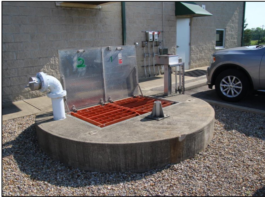
Figure 2-16: Effluent Pump Station
