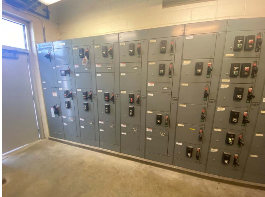
Figure 11: MCC-PO in Post Treatment Building Electrical Room
