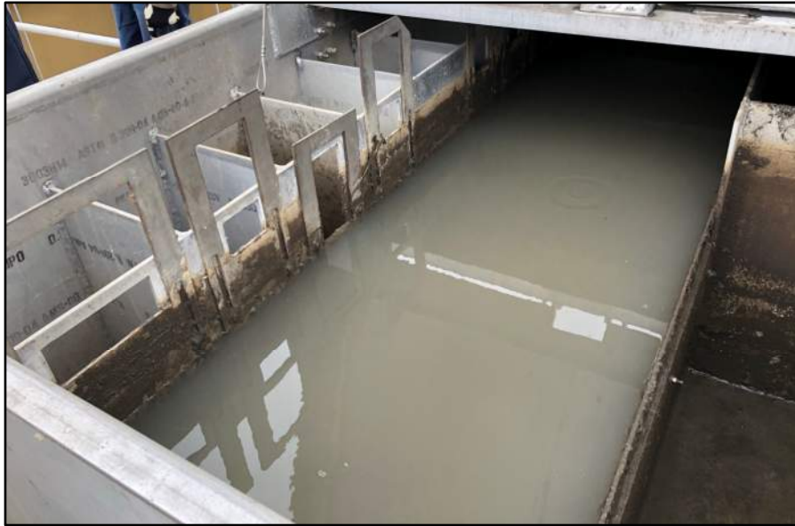
Figure 2-4. Influent Distribution Box
