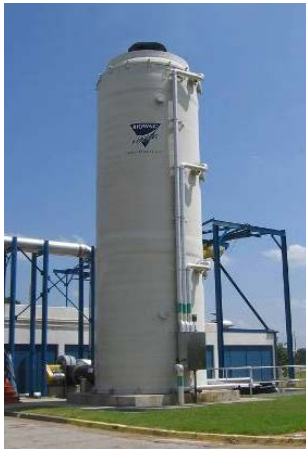
Figure 3-4 Representative Biotrickling Filter
