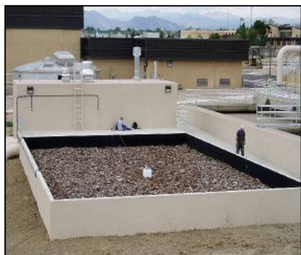
Figure 3-3 Representative Biofilter Unit
