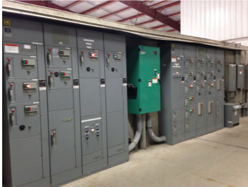
Figure 15: Electrical Equipment without Isolation from Wastewater Treatment System
