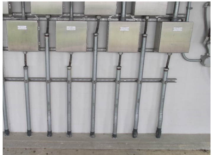
Photo 29: Lower Scioto WRF - Scum Pump Terminal Box
