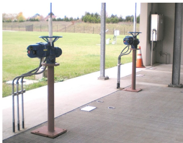
Photo 28: Lower Scioto WRF - Processing Pump Station
