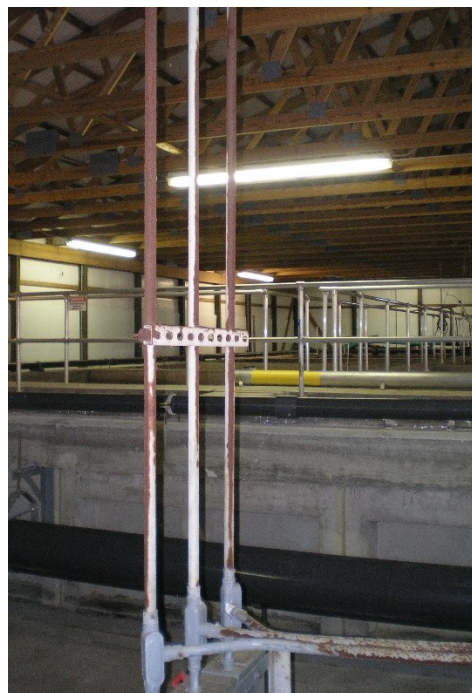
Photo 23: Tartan - Conduits at RAS Well
