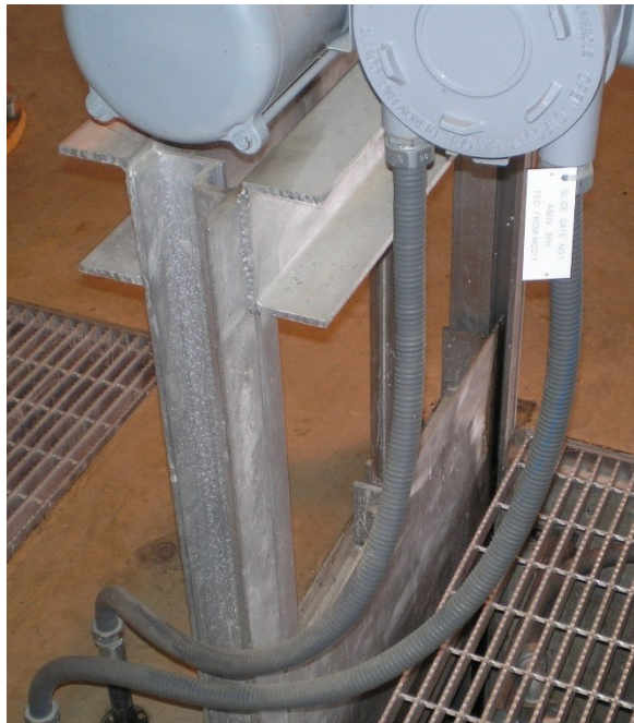
Photo 24: Lower Scioto WRF - Actuator in Screenings
