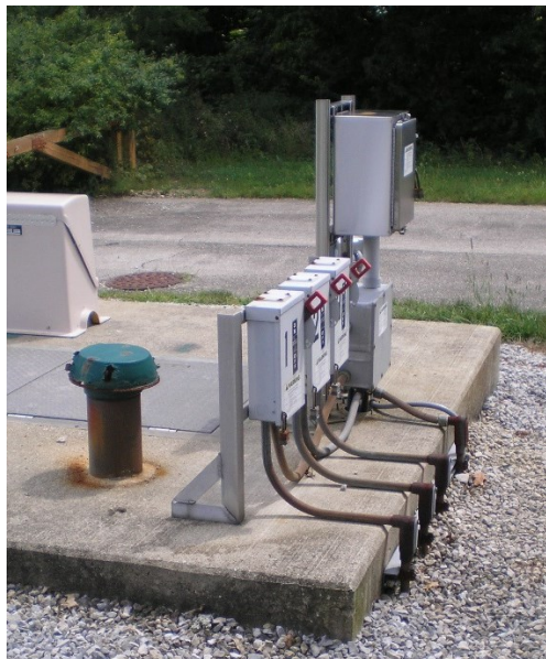
Photo 22: Tartan - Influent Pump Station
