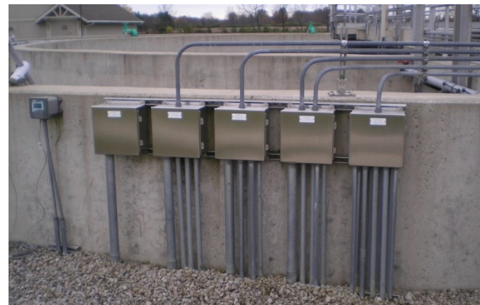
Photo 27: Lower Scioto WRF - Aeration/Clarifier
